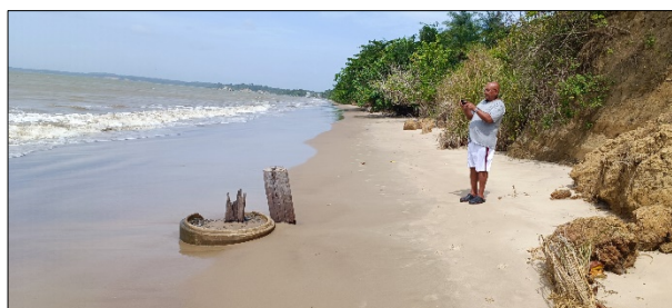
Photo 48. Outcrop of old structures due to sand loss.
