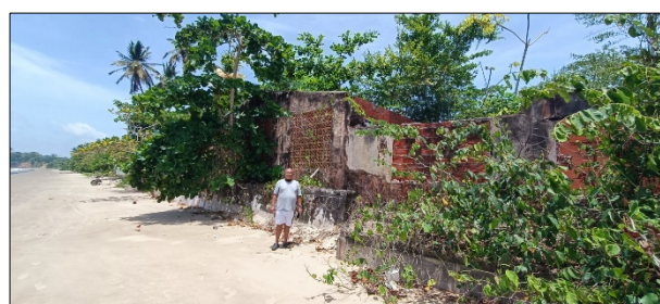
Photo 38. Abandoned house and protection wall on the beach.
