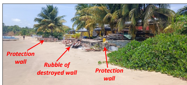
Photo 37. Protection walls and buildings on the beach and rubble from their destruction by the wave.
